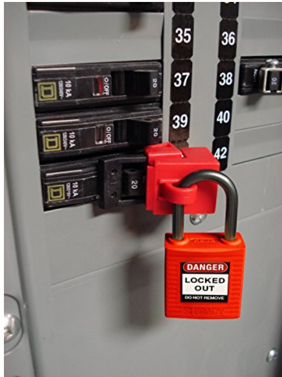
Figure 1.5: Always lockout main panel circuit breakers and ensure two line breaks between the point of connection and the source (open-points)
